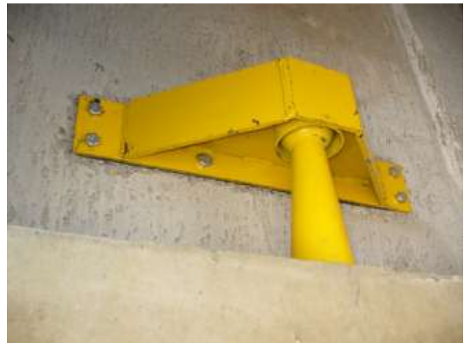
Figure 13. Damper used in the bridge in Sorocayense
